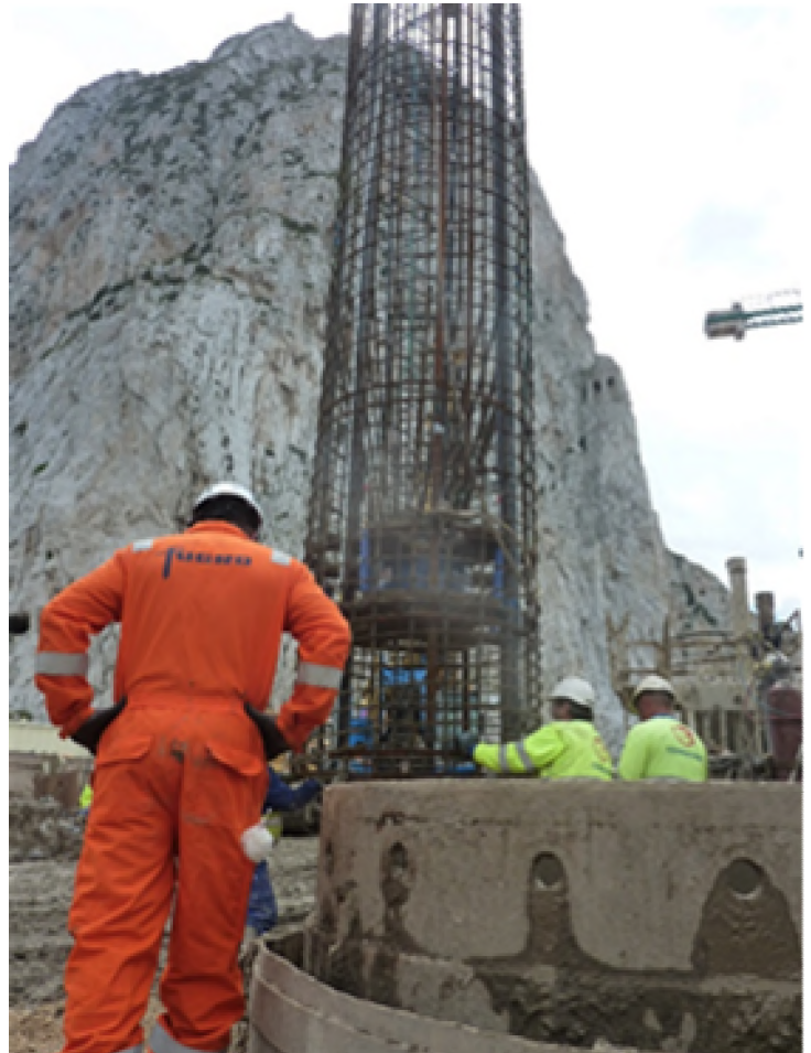
Reinforcing cage, O-cell® and instrumentation ready for installation into the pile bore
